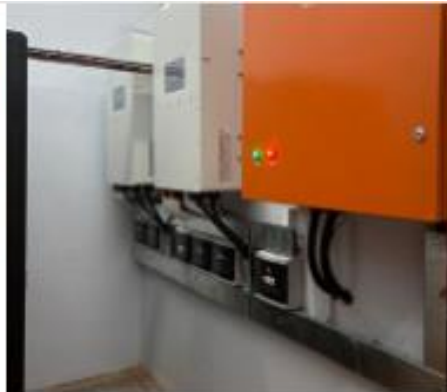
GROVE PRIMARY, CLAREMONT 100kW Deye HV with 102kWh Sunwoda HV Lithium and 25.5kWp Solar PV 2024
