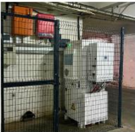
79 ROELAND, CAPE TOWN 50kW Deye HV with Sunwoda HV Energy Station, 25kW Goodwe Grid-Tie and 75kWp Solar PV 2024
