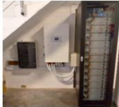
LONDON RD, BRACKENFELL 49.5kWp with 50kW Deye HV & 62kWh Deye Lithium 2023
