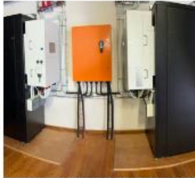
CLAREDON SCHOOL, EAST LONDON 100kW Deye HV with 200kWh Deye HV Lithium 2023
