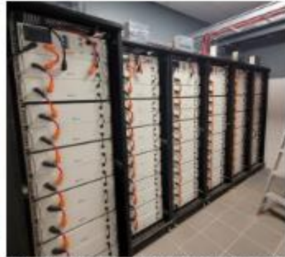
REDDAM COLLEGE, DURBANVILLE 150kW Deye HV with 360kWh Deye HV Lithium 2023
