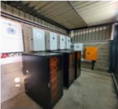
GLC DEVELOPMENTS, DURBANVILLE 64.2kWp with 96kW Sunsynk Hybrid & 102kWh Revov Lithium 2023
