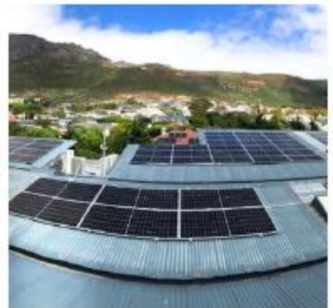
MILTON'S WAY, STEENBERG 100kW Deye HV with 102kWh Sunwoda HV Lithium and 62.1kWp Solar PV 2024
