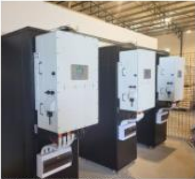
AFRIKELP, CAPE TOWN 150kW Deye HV with 184kWh Deye HV Lithium 2023
