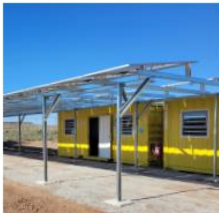
GAMMA CAMP, NORTHERN CAPE 50kW Deye HV with 63kWh Sunwoda HV Lithium and 29.3kWp Solar PV 2024
