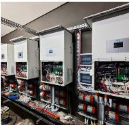
VREDENBERG MALL 250kW Deye HV with 307kWh Sunwoda HV Lithium 2024
