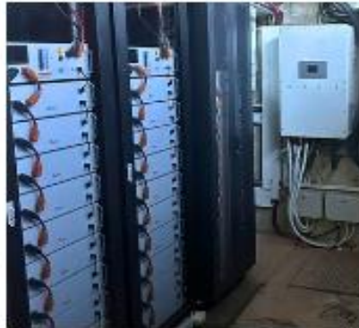
BP GARAGE, FRANSCHOEK 73kWp with 100kW Deye HV & 194kWh Deye Lithium 2023
